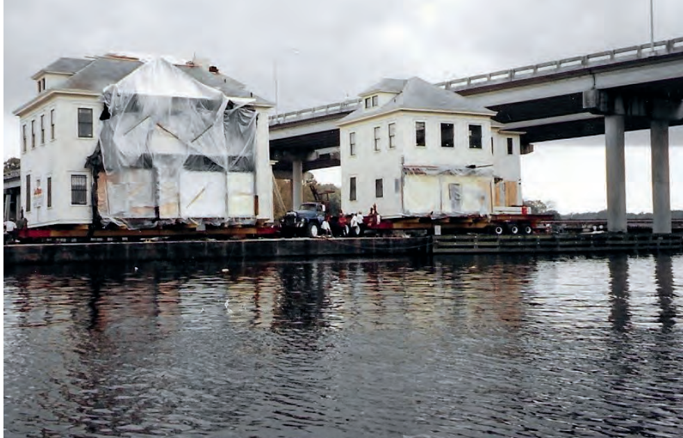
The Victorian house where Reinsch lived as a child was uprooted and split in half so it could travel to its new home on a plot of land along the Cedar River in Jacksonville, Florida.
